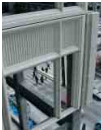
This construction photo shows the delicate detail made possible by the use of GFRC panels.
